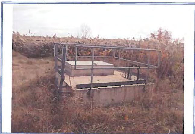
Station de pompage (ne sert plus)
