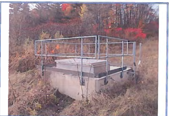
Station de pompage (ne sert plus)
